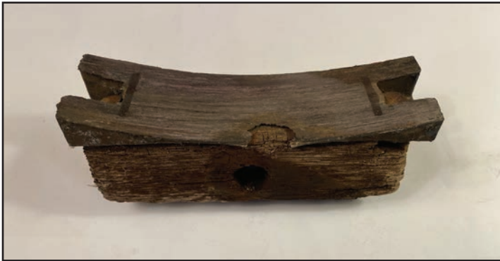
This brake block and liner have reached the end of their useful life and should be replaced
